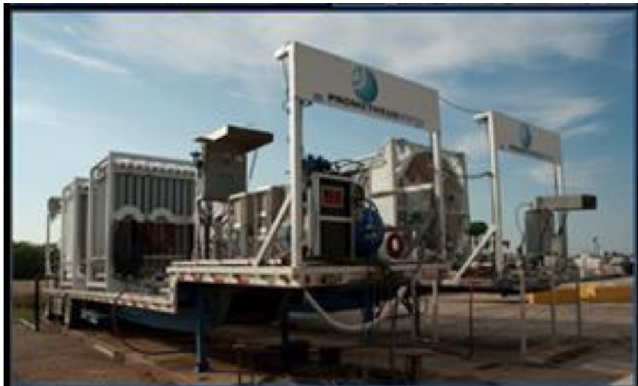
Figure 18-4. Example of LNG Powered Reciprocating Piston Engine Generator
